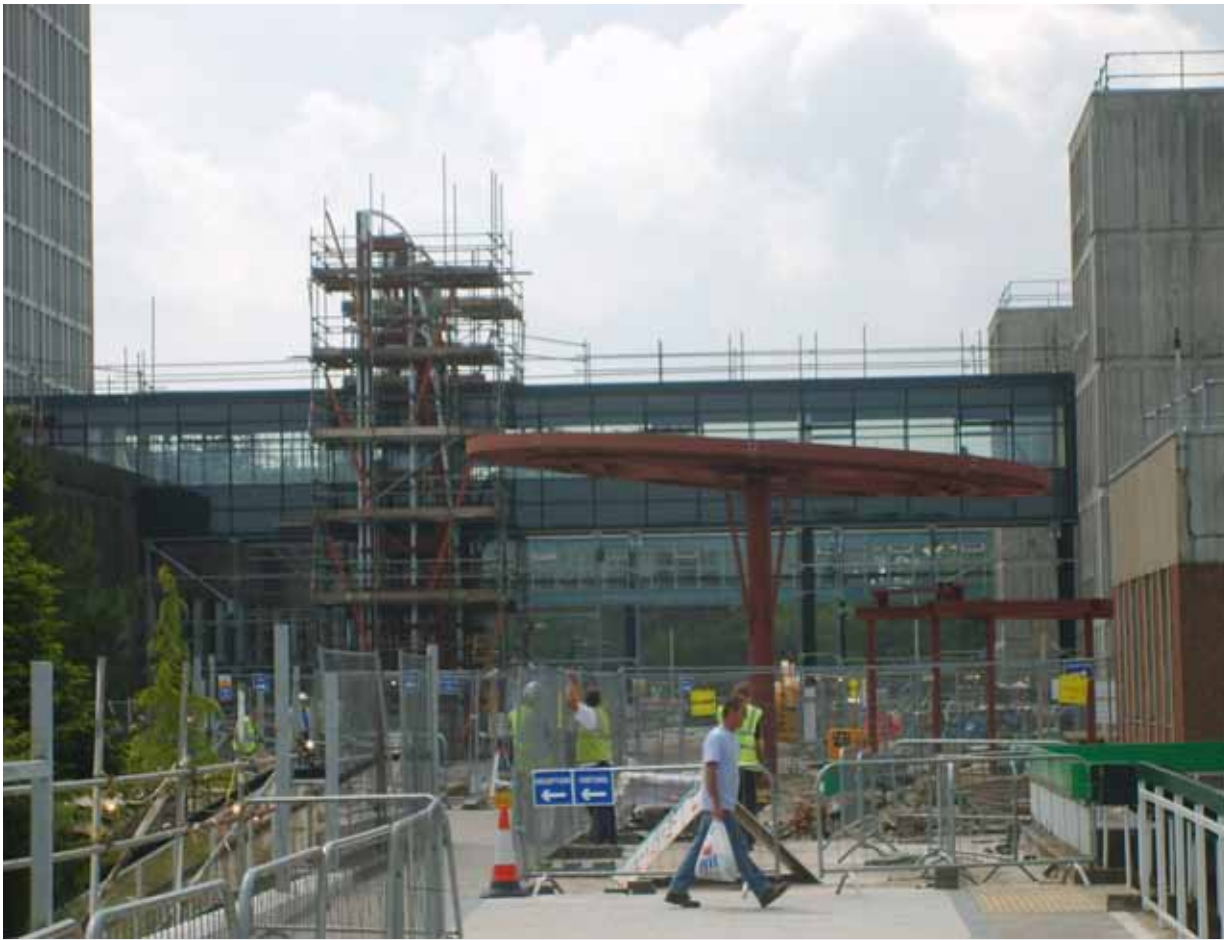
This building project in Swansea, South-Wales, complies with the UK government policy on sustainable timber procurement.
